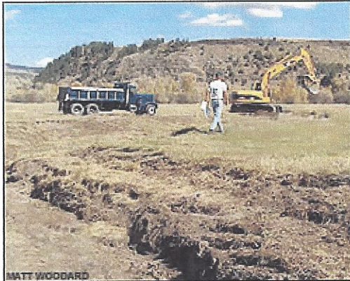
MATT WOODARD Trout Unlimited stream design specialist, Jim MacCartney, oversees the construction of Garden Creek's new channel.
